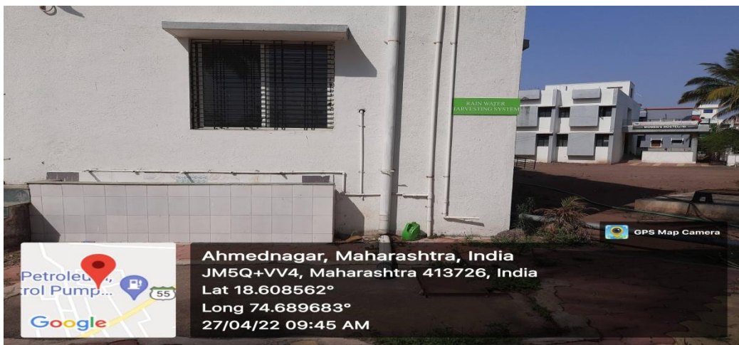
Rain water Harvesting System
